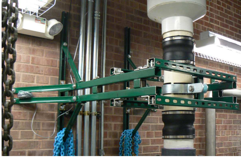
FIG. 5: The vibration-damping system on our 2000 m 3 /h Roots blower. A section of 6 in. PVC pipe is suspended between two rubber couplers. A riser clamp is attached to the pipe (with rubber), and is attached to a support structure rigidly coupled to the wall. All bolts are fastened with rubber washers for additional vibration damping. The support structure minimizes displacement of the pipe section, which reduces the amount of vibration coupled into the pumpline through the upper rubber coupler.
